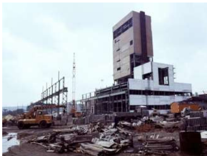
Figure 67 – Construction of the main building in 1977 during the transformation of the production mine into a disposal facility from 1974 to 1978 [105]
