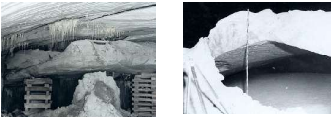
Figure 71 – Loose rocks and drip points in mining chamber 5 at the 700-metre level (1993) and arching of the ground in mining chamber 6 at the 553-metre level (1967) [114]
