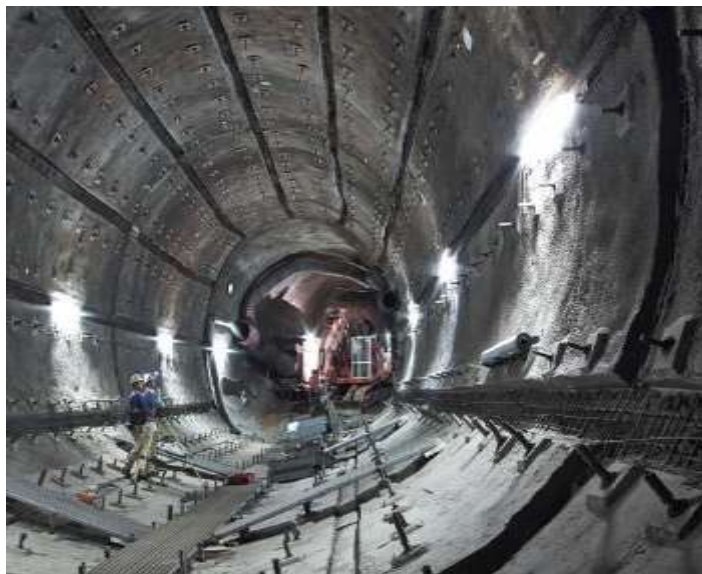
Figure 66 – Extension of the emplacement transport section as a tunnel tube (connection of the Konrad 2 shaft with the emplacement chambers) [102]
