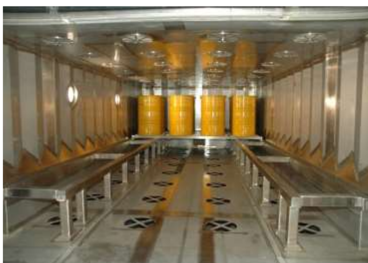
Figure 17 – Drum drying facility
