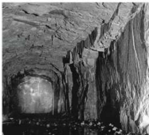
Figure 43 – Large shear strain can give the rock mass strongly anisotropic hydraulic and mechanical properties [85].
