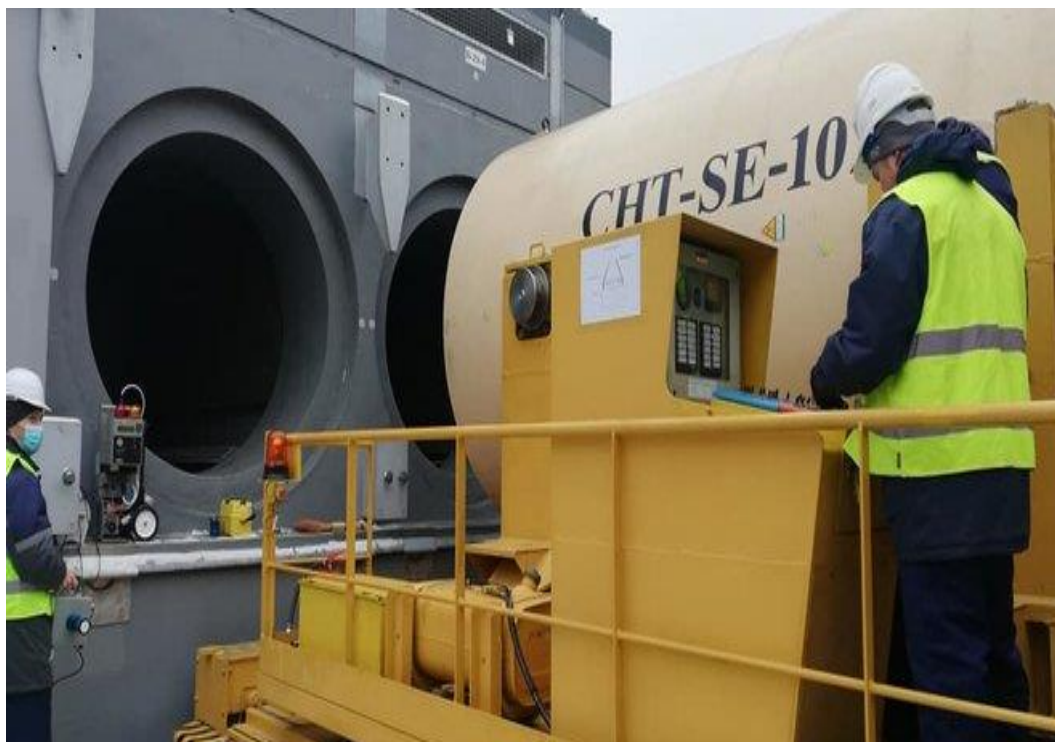
Figure 19 – Loading of the first DWC with SNF into ISF-2 concrete storage module #2 (CSM – 2).
