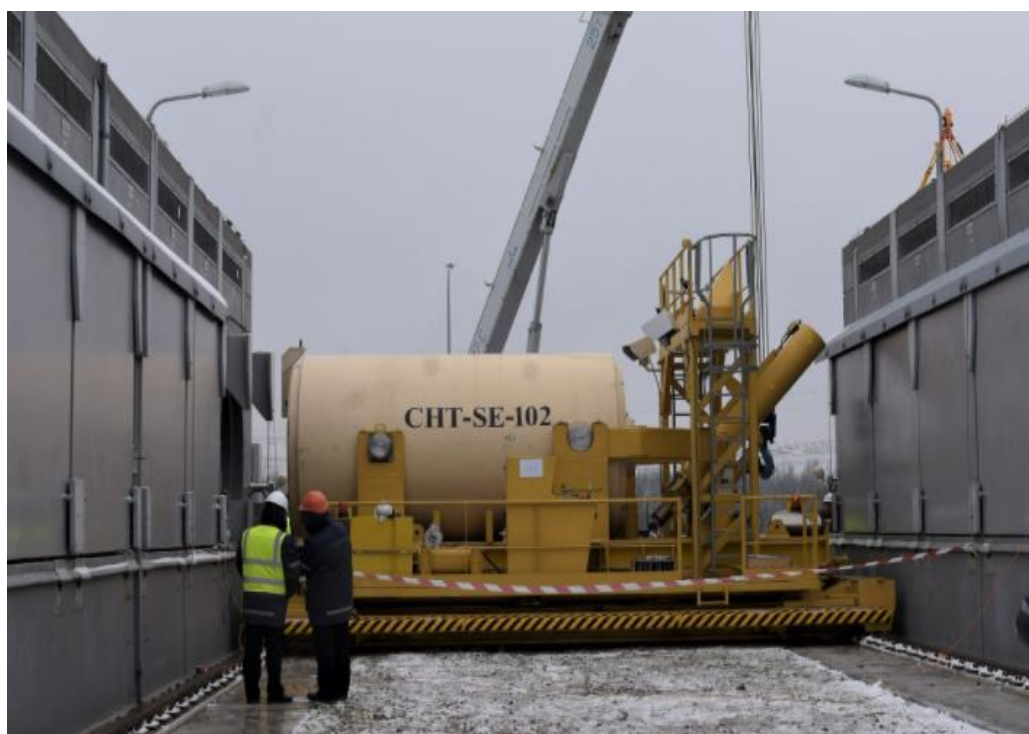
Figure 18 – Loading of the first DWC with SNF into ISF-2 concrete storage module #1 (CSM -1).
