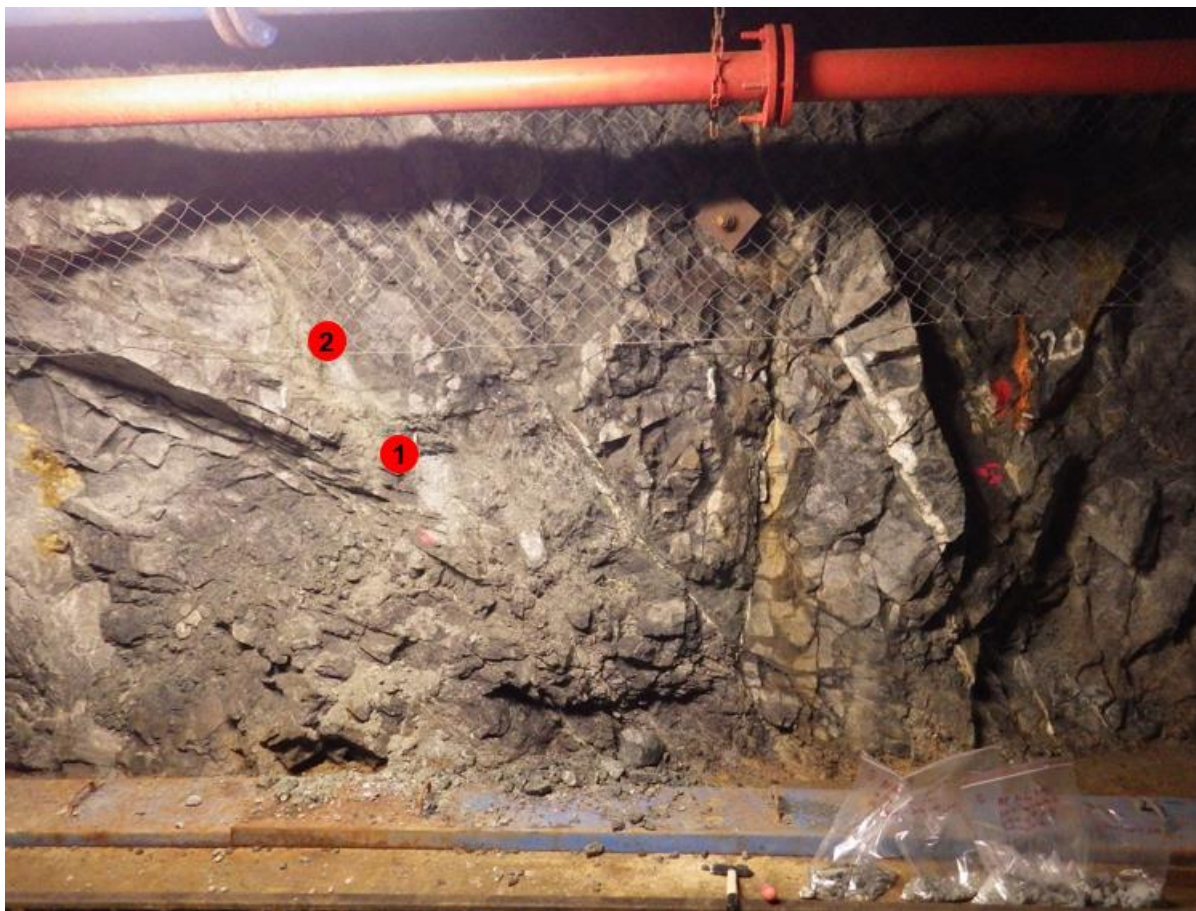
Figure 1-10 Fracture with chloritic infill material located in the corridor BZ-XIIJ (chainage 218 m) with indicated sampling sites (red circles 1 and 2)
