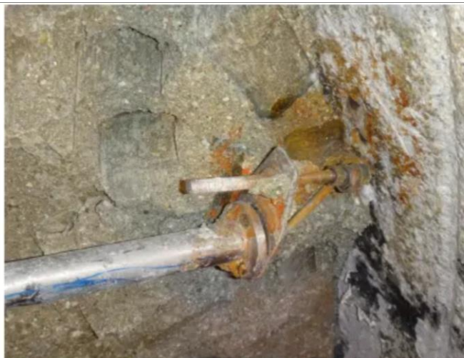
Figure 15 Photograph showing corrosion areas on and in the vicinity of an extensometer anchorage used in the FEBEX experiment (García-Siñeriz et al., 2016).
