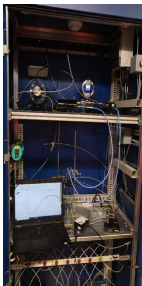
Figure 105: Experimental setup of the optical pH sensor prototype in the ACA cabinet located in the GED gallery in Bure
