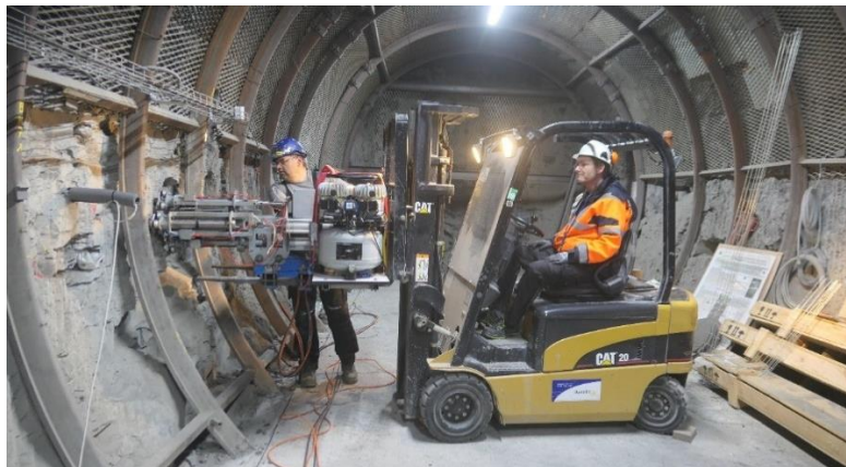
Figure 35: Magnetostrictive vibration system applied on the side wall of Gallery East-03. The source is equipped with four magnetostrictive actuators which work simultaneously using a real-time control system.
