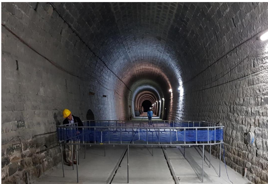
Figure 7-7: Prototype wireless antenna installed in the Tournemire URL (France) as part of Modern2020 [17]
