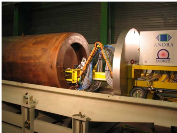
Figure 16: View Showing Emplacement Cart, Radiation Shield, Pushing Jack, Canister and Gripping Mechanism
