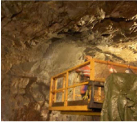
Figure 20: Field test with low-pH shotcrete for rock support at Äspö HRL, Sweden
