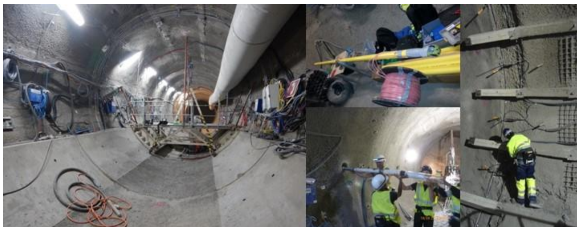
Figure 16 Installation of sensors in boreholes, shotcrete and poured concrete in GER gallery
