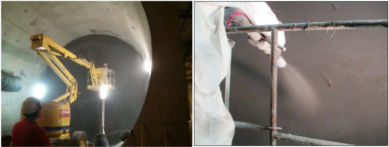
Figure 4.4: Installing the second containment wall made of low pH shotcrete in FSS.
