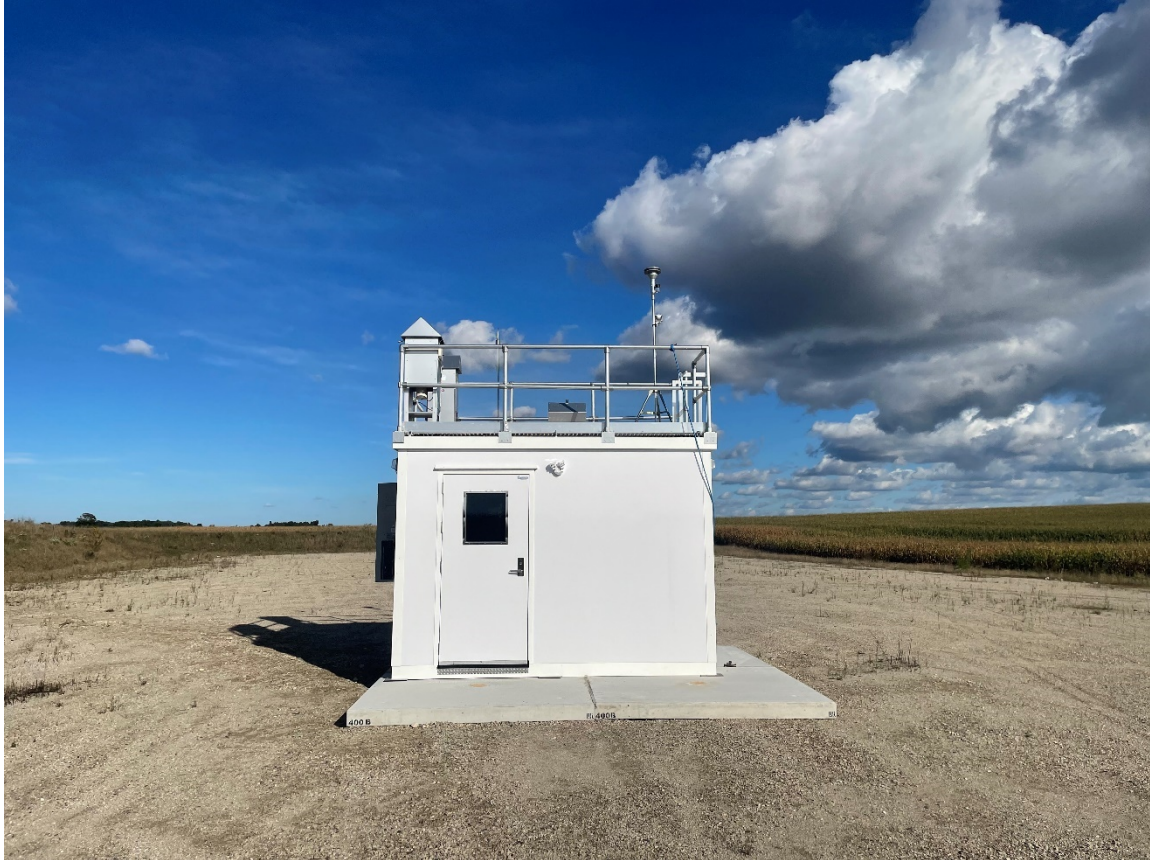
Figure 7-8: Atmospheric Monitoring Station at Borehole 1
