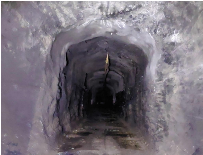
The first 5 deposition tunnels are excavated and as part of commissioning the Trial Run of Final Disposal takes places in as tunnel (in figure) beside the disposal area
