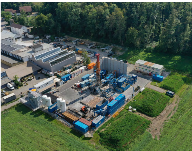
Drone photo of the drilling site in Bülach after setting up the drilling rig ( nagra.ch )
