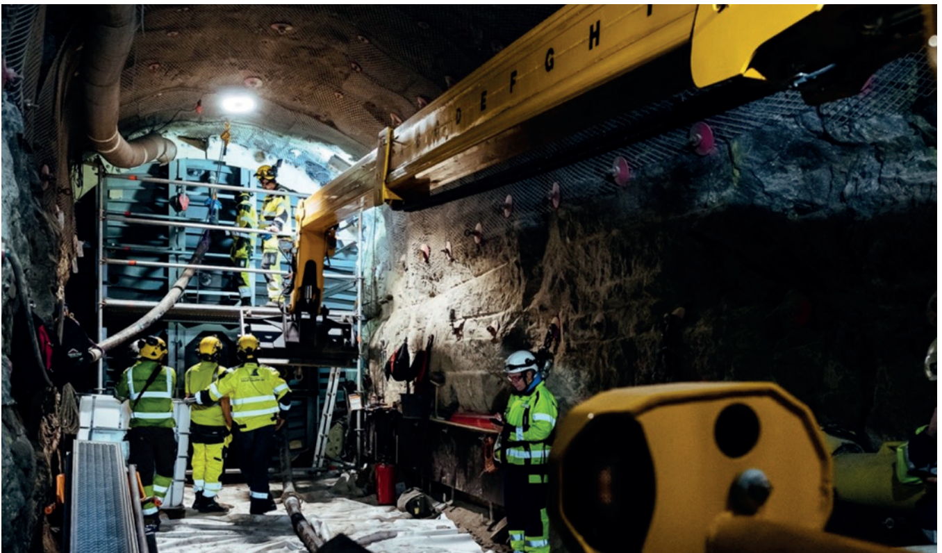
Casting of the end plug of the Full-scale In-situ System Test, photo Posiva Oy
