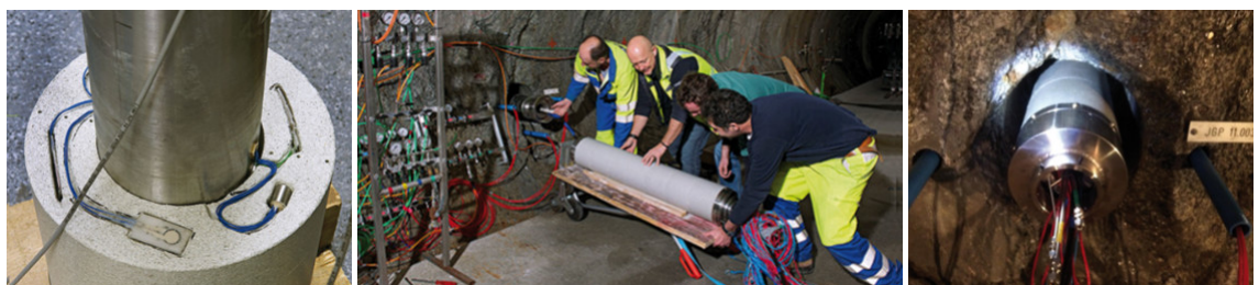
Fig. 5: CFM i-BET source assembly (bentonite rings and sensors, left) and installation at the experiment site (centre & right).
